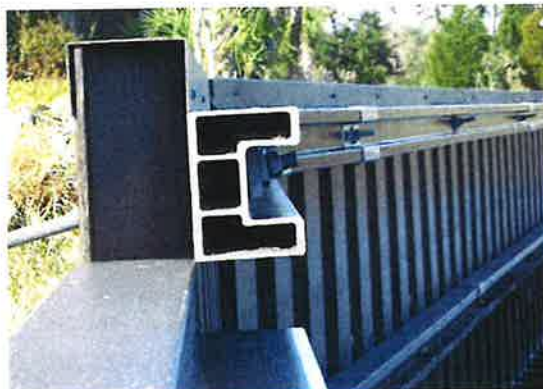
Example of composite bulkhead, wale, and cap with hot dipped anchor tie rods.
